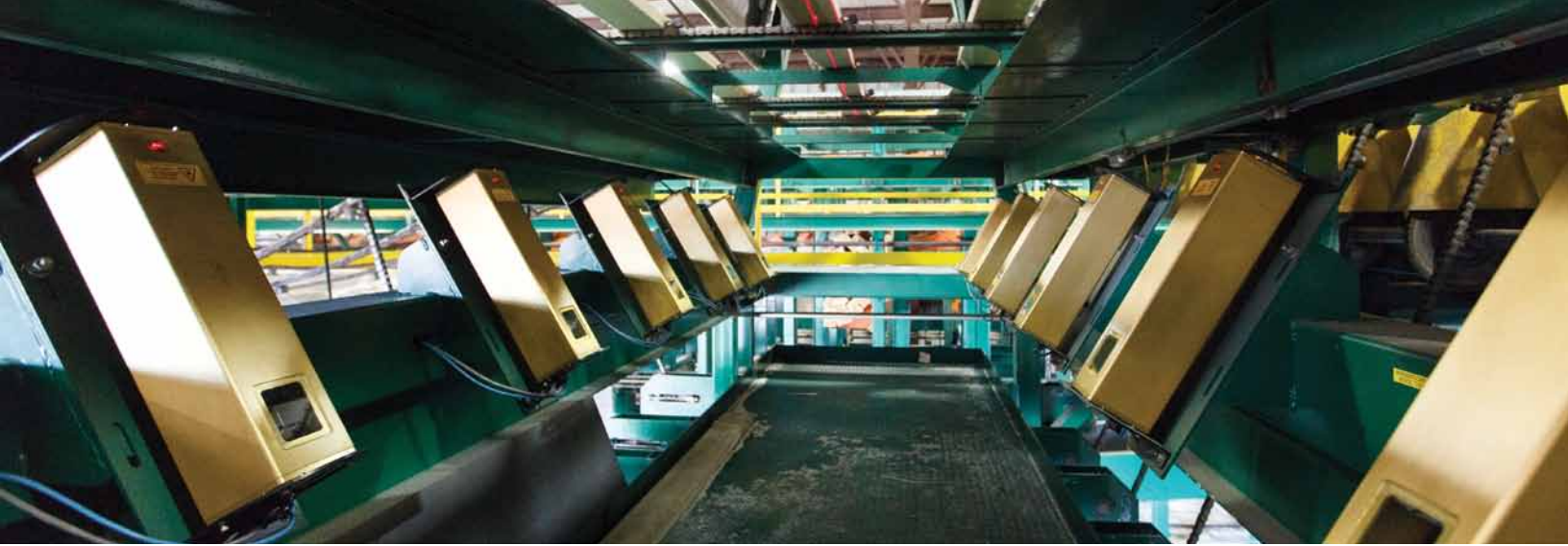
JoeScan scan heads transversely profile boards in the trimmer.
